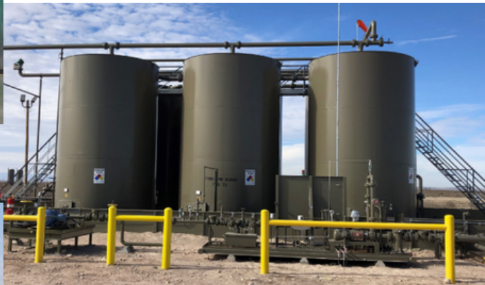
Tank battery installation. +12 months after installation and looks like new.
